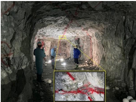
An adit excavated as part of the geological survey. At the ceiling near the dead end, the location of the centre of the Hyper-Kamiokande dome is marked (inset photo).
