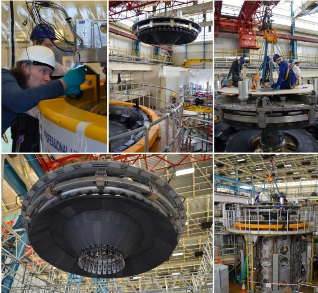
The installation of the MAST-U upper end plate which was craned into place in November and marks a major milestone in the MAST-U project.
